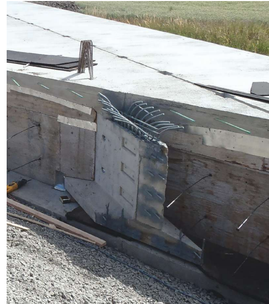
Skewed decked bulb-tee girders erected for the Hatley Bridge, Whitman County, Wash. Photo: Whitman County Public Works Department.
