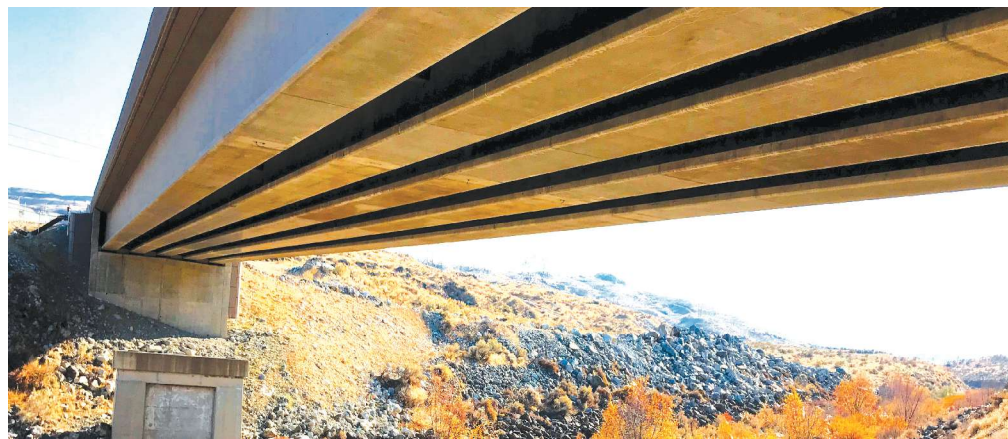
View of completed bridge from below. Piers from existing bridge remain, which were used to support girder segments at splice locations.
