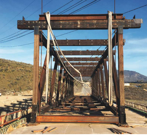
The existing truss bridge was lifted onto the completed superstructure and dismantled.
