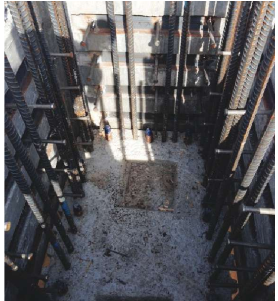
Steel channels with welded studs form shear keys as part of the column-to-cap connection. Photo: Modjeski and Masters.
