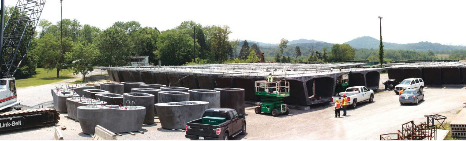
Pier and superstructure segments for Bridge 2 in the precast concrete yard. Photo: Eastern Federal Lands Highway Division of the Federal Highway Administration.
