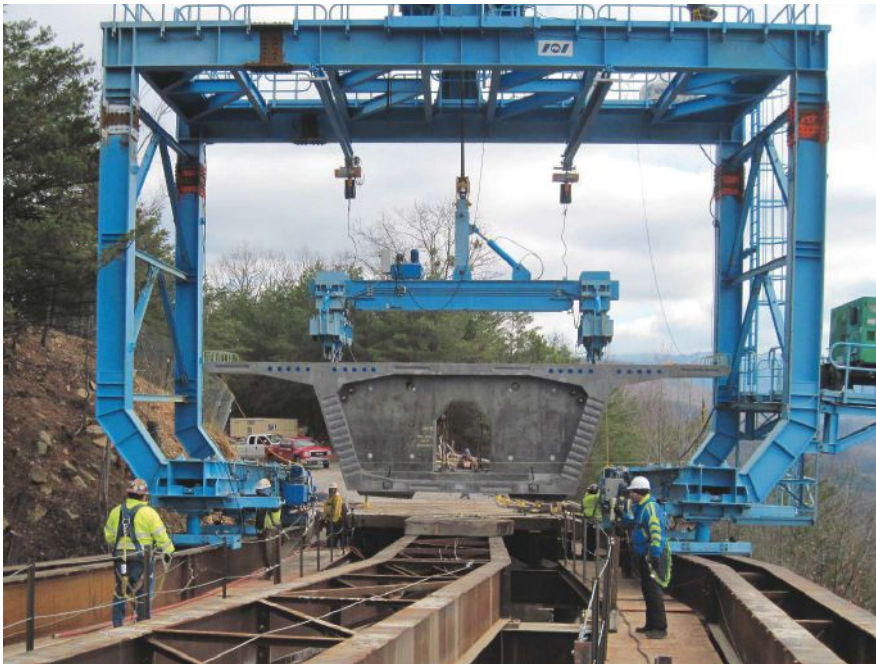
Due to the steep terrain at the site for Bridge 2, a temporary trestle/falsework system was constructed to support a gantry crane to erect the precast concrete segments. The gantry is lifting a pier segment in this photo. The access hole in the segment is visible. Photo: Eastern Federal Lands Highway Division of the Federal Highway Administration.
