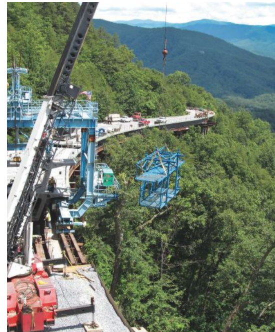
Segment erection as Bridge 2 nears completion. Photo: Great Smoky Mountains National Park, National Park Service.
