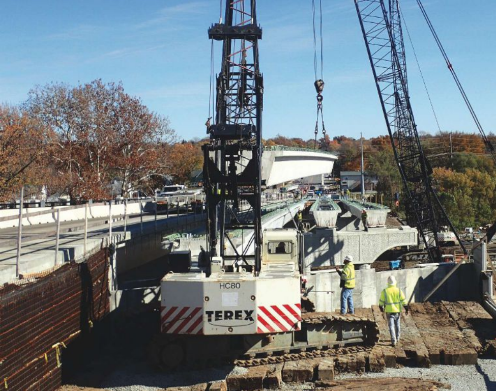
Prestressed concrete U-beams being erected at abutment number 1. The crane is sitting on crane pads within the mechanically stabilized earth fill. Photo: United Consulting.
