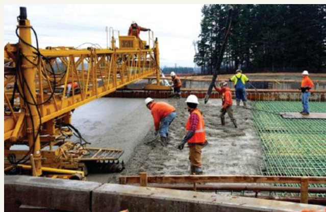
Figure 3. Use of epoxy-coated reinforcement to protect the bridge deck from corrosion-induced damage.
