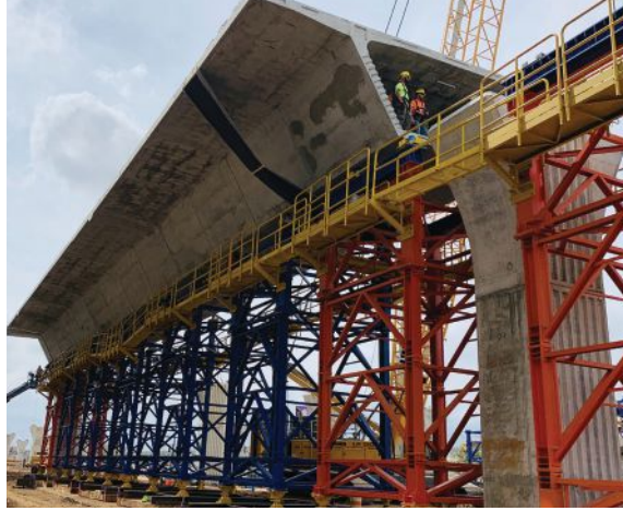
The erection of the first span was completed on March 11, 2019. The main elements of the shoring towers were color coded to be easily identified by field crews for their proper locations. Approximately 127 individual shoring towers were provided, which allowed concurrent work on up to eight fronts. Photo: Structural Technologies.
