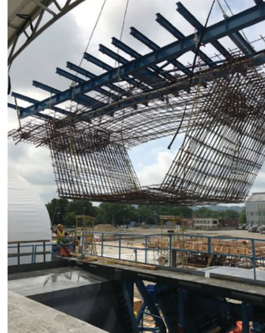
Reinforcing bar cage with transverse tendons being installed into forms. Photo: Johnson Bros.
