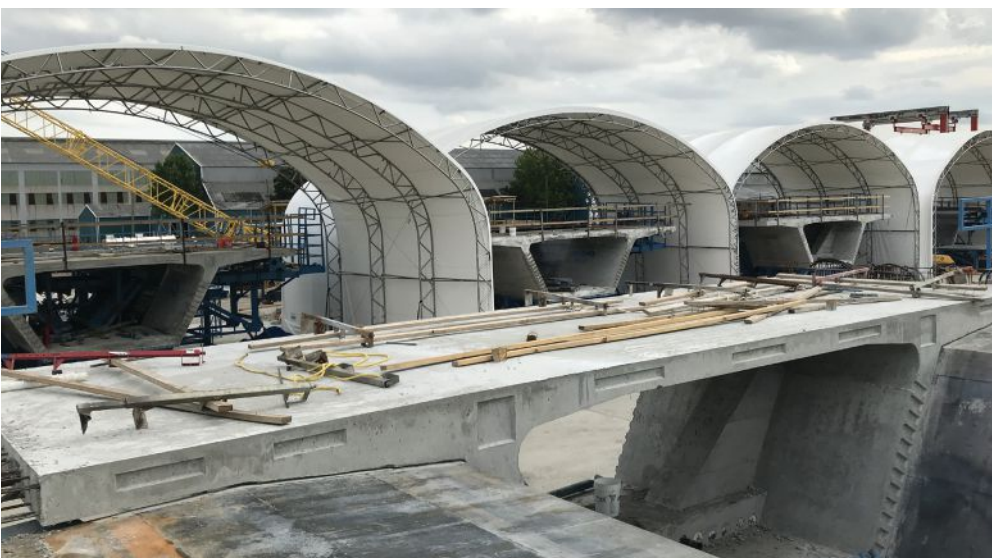
Casting cells for precast concrete box-girder segments with protective covers. Photo: Johnson Bros.
