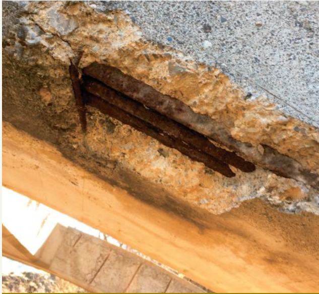
Although concrete spalling and corrosion of the reinforcement were widespread on the concrete arch, the reinforcement maintained its integrity, leading to the decision to rehabilitate rather than replace the bridge. Photo: Rebecca Burrow.
