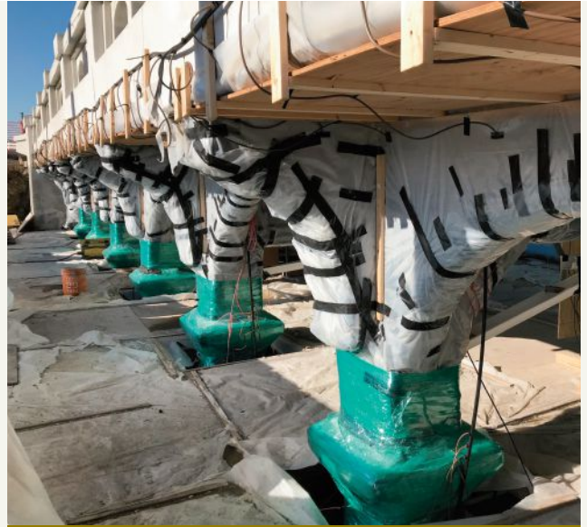
The realkalization system involved wrapping the bridge with insulation matting to store the electrolyte, folding titanium mesh over that, and containing the system with a plastic covering. Photo: Rebecca Burrow.
