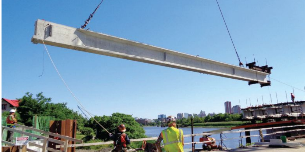
Erection of an end girder segment in span 1 from the working platform. Note the preinstalled strongback at the pier end of the segment and the end block for post-tensioning anchorages at the abutment end of the segment. The end detail of the girders at the abutments was modified at the request of the precaster because, in their experience, the small piece of the top flange that extends beyond the end block has a tendency to crack at the interface. Photo: R.E. Pierson Construction Company.
