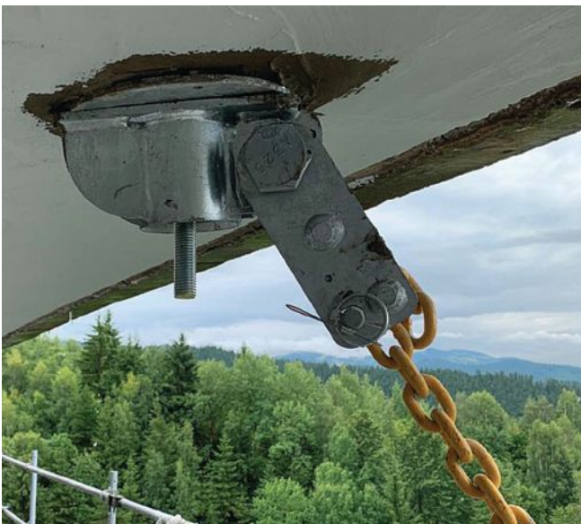
Figure 4. An innovative proprietary rotating-suspension-point assembly was used for the rehabilitation of the Caraçu Viaduct in Romania. Photo: Doug Knapp.
