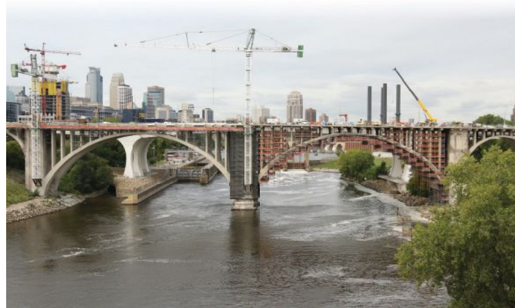
Figure 1. View of spans 3 to 6 of the Tenth Avenue Bridge in Minneapolis, Minn., looking north. Suspended platforms were used as debris shields on span 4 and for work access on span 5. Photo: Doug Knapp.
