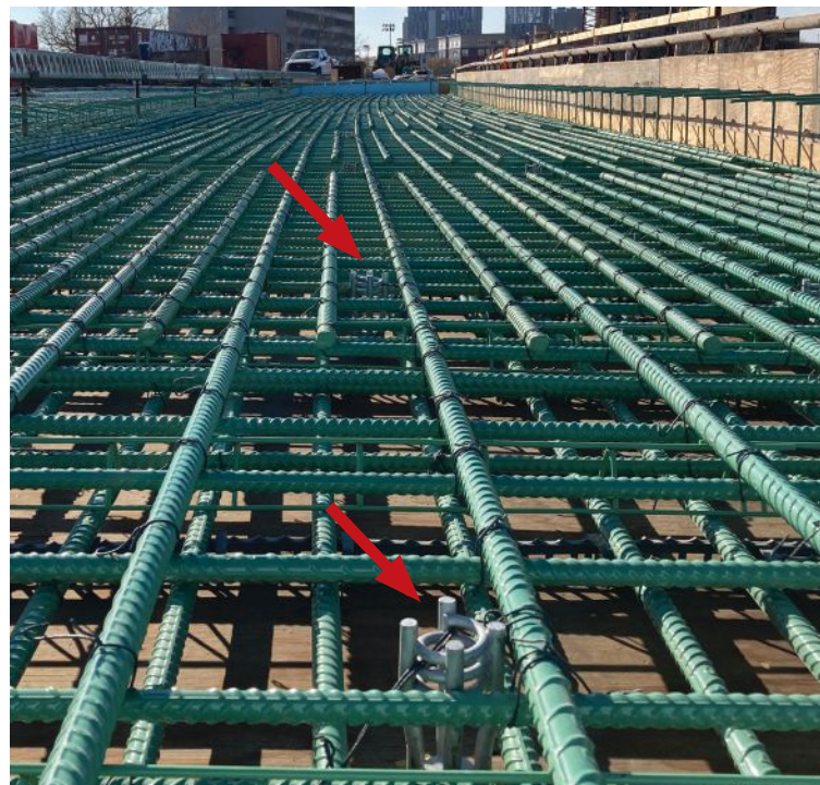
Figure 2. Embedded concrete inserts (indicated with arrows) are secured to the deck slab reinforcement with wire ties before placement of the new Tenth Avenue Bridge deck. Photo: Doug Knapp.
