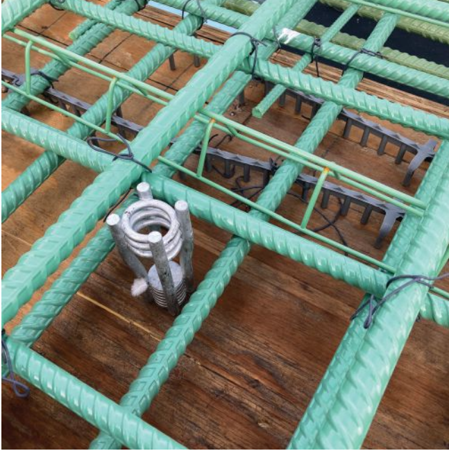
Figure 3. Using hundreds of embedded concrete inserts in the cast-in-place bridge deck eliminated hundreds of hours of labor to drill holes for post-installed anchors. Photo: Doug Knapp.
