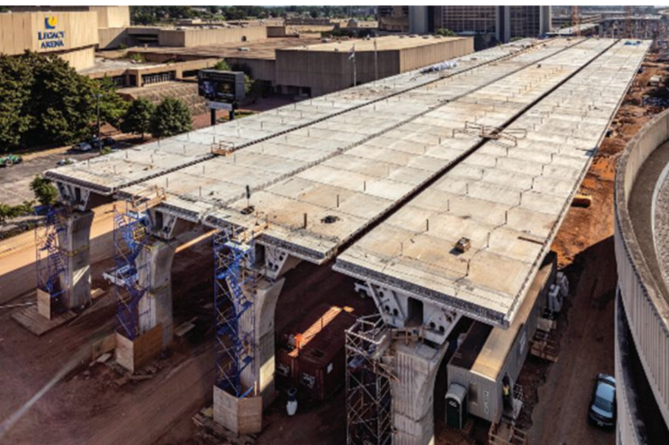
Load rating of the new 172-span, 1 million ft 2 structure for the Interstate 20/Interstate 59 Central Business District Bridges in Birmingham, Ala., required over 160,000 individual rating evaluations. Photo: Volkert Inc.
