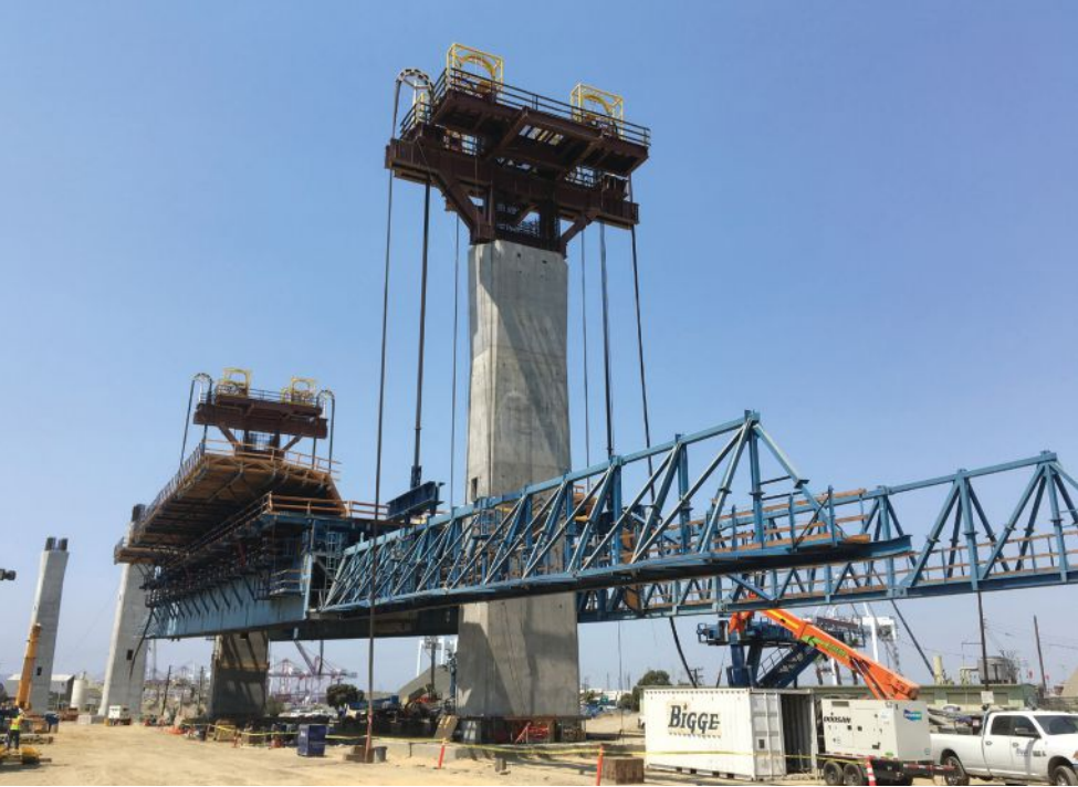
The movable scaffold system (MSS) being lifted by strand jacks. The brackets, one of which can be seen in the background on the right below the MSS, were raised in a separate operation. The MSS center section was a heavy box girder that supported the concrete span and lighter trusses at each end for launching. The total length of the MSS was over 500 ft. Photo: SFI.
