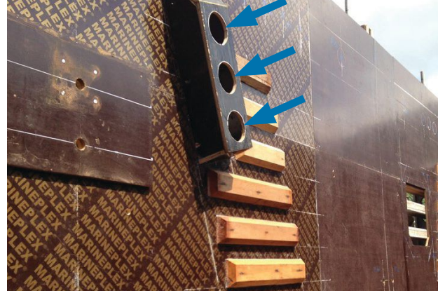
Figure 4. Formwork for the face of the CIP straddle beam where additional tolerance has been created by placing blockouts around post-tensioning ducts where they enter a wet joint (ducts will be installed in holes in blockout, indicated with arrows). The blockout increases the length of the ducts crossing the splice, adding flexibility to connect the ducts to the precast concrete segment.
