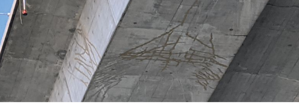
Figure 3. Epoxy-injected cracks in the West Seattle Bridge (2020). Photo: John Stanton.
