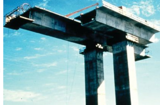
The precast concrete segments were erected using balanced-cantilever construction. A custom-designed erection jig was used to hold a segment in place for application of the joint epoxy to the mating faces is visible. Photo: Alan Matejowsky.
