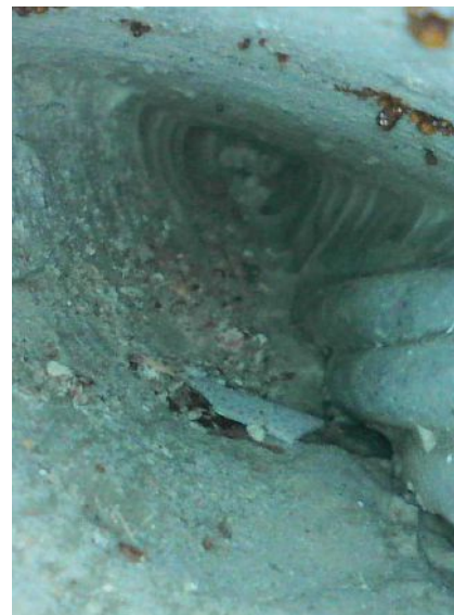
Borescope image of small void in deck tendon near post-tensioning anchor.
