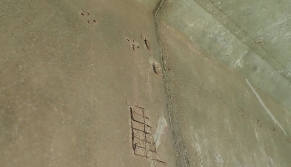
Spalling on the exterior face of the box girder exposed corroded supplemental (not indicated in original plans) wire-mesh reinforcement with insufficient clear cover. Photo: Wiss, Janney, Elstner Associates Inc.
