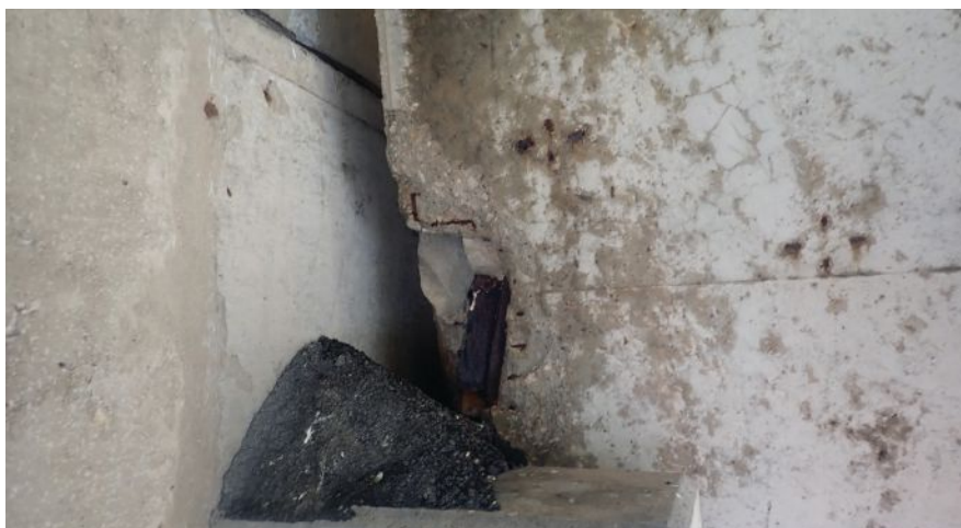
Moderate corrosion of continuity tendon anchor at end of box girder.
