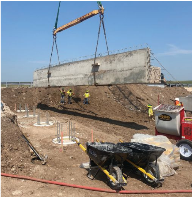
Setting a precast concrete abutment on the drilled-shaft foundations. Reinforcement extending from drilled shafts fits into ducts in the precast concrete cap, which are then grouted.
