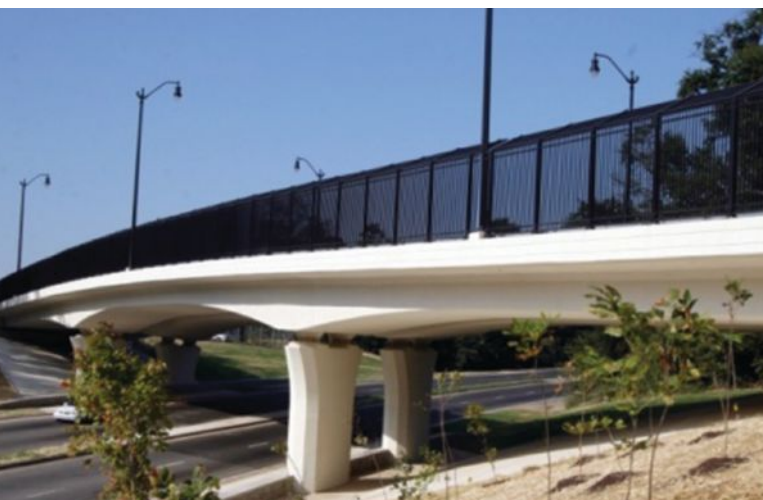
The Southern Avenue Bridge over Suitland Parkway is a three-span, 413-ft-long cast-in-place concrete, post-tensioned, haunched box-girder structure. Photo: CDM Smith.
