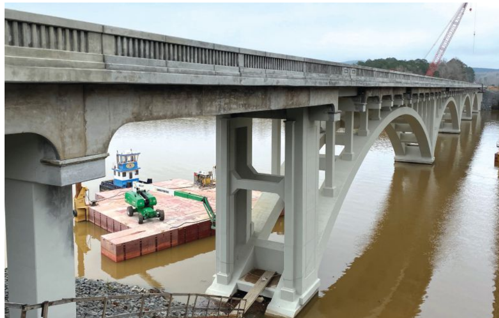
Precast concrete fascia panels were used to preserve the historic aesthetics of the original arch structure.
