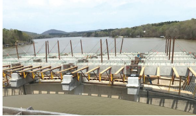
Prestressed concrete box beams are placed and await the cast-in-place concrete continuity diaphragms.
