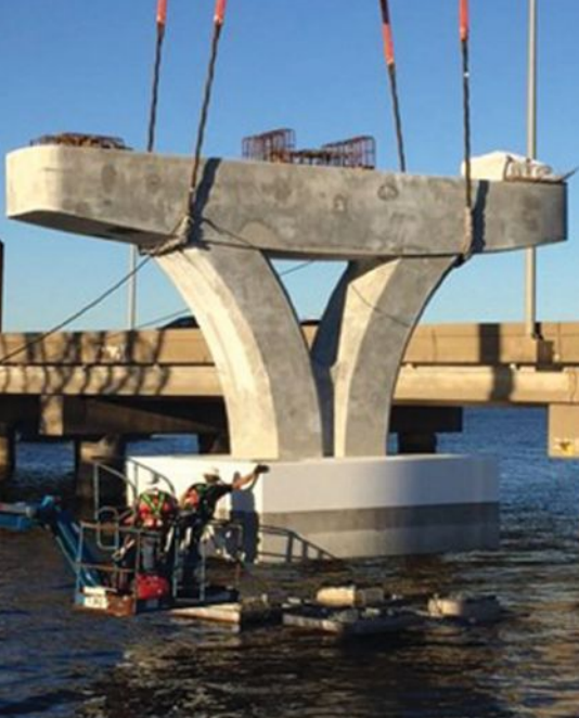
Workers set a shorter V-pier unit, for which the cap, column, and footing were precast as a unit. Photo: WSP USA.
