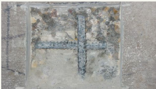
Figure 3. Concrete repair area ready for repair with square edge geometry, saw-cut edges, and properly cleaned and exposed reinforcement. Photo: Vector Construction.
