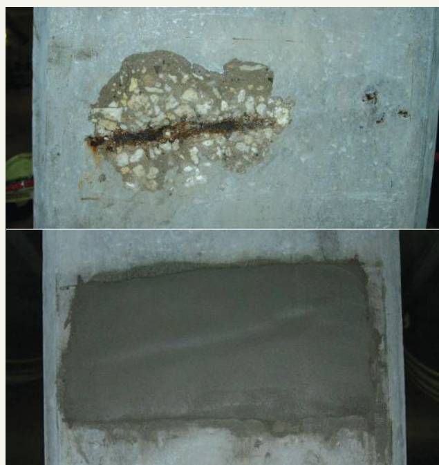
Figure 5. Before-and-after photos of a concrete repair are recommended as part of a quality control program. Photos: Vector Construction.
