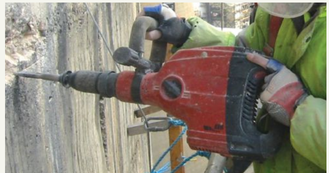
Figure 2. Concrete is prepared for repair by removing deteriorated concrete using a small chipping hammer. Photo: American Concrete Institute Repair Application Procedure (RAP) Bulletin 6.
