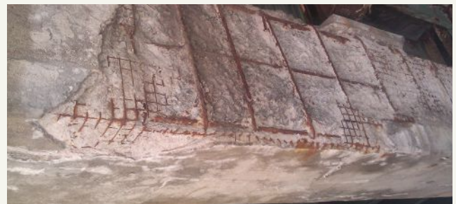
Figure 1. Failed shotcrete repair on a bridge pier cap. Photo: Vector Corrosion Technologies.
