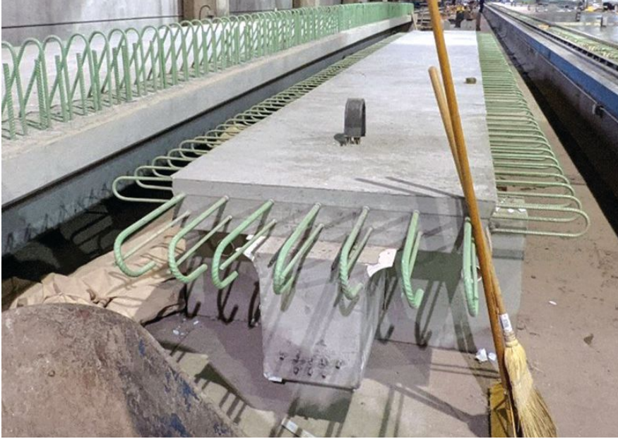
Single-stem Northeast Extreme Tee D beam after curing and before end diaphragm placement. Epoxy-coated mild reinforcement extending from the top flanges will become part of the cast-in-place concrete closure pours and end diaphragm.
