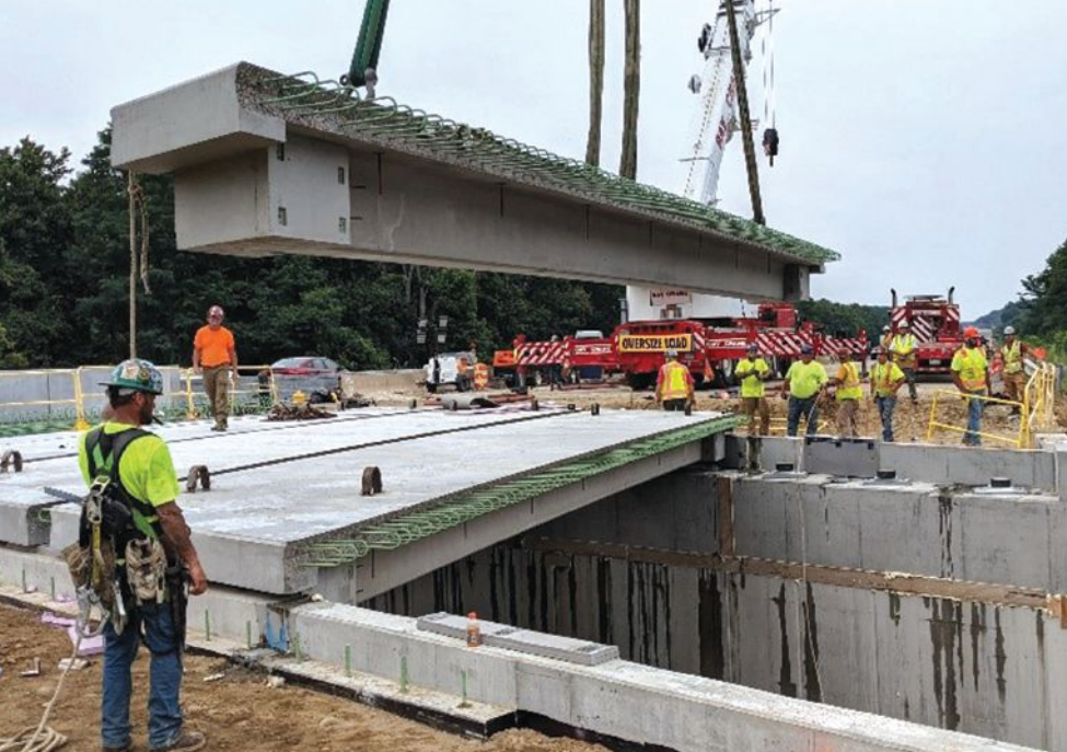
Northeast Extreme Tee D beams were typically placed late on Saturday afternoon during the weekend closure. A single-tee beam is being erected in this photo.
