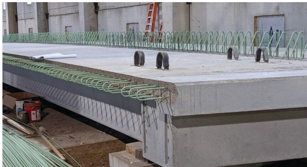
A double-stem Northeast Extreme Tee D beam after end diaphragm placement in a secondary pour. Reinforcement for the barrier is visible at the far edge of the deck slab.
