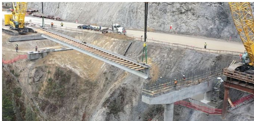
Erecting an exterior girder with preinstalled overhang brackets for the Kicking Horse Canyon project, Phase 4, in Golden, BC, Canada. Because the preinstalled overhang brackets impose vertical and torsional construction loads on the exterior girder, lateral stability of the girder must be investigated while the girder is supported by cranes and after it is set on bearings.
