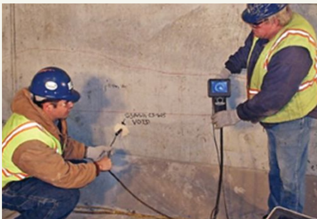
Inspection of a void in a grouted post-tensioning duct using a borescope. Photo: Structural Technologies.
