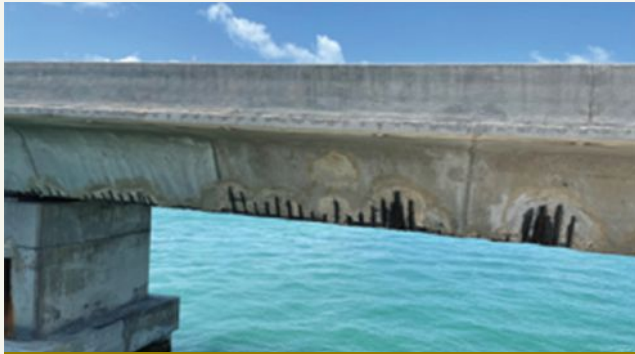
A precast concrete segmental bridge with loss of concrete cover and reinforcement cross-sectional area due to corrosion of reinforcement after approximately 45 years of service and exposure to a saltwater environment. Photo: Finley Engineering Group.
