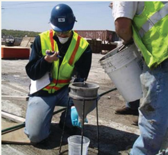
Post-tensioning system details and procedures, quality assessment, quality control, and technician training and certification requirements have all contributed to more successful and reliable tendon grouting. Photo: Structural Technologies.
