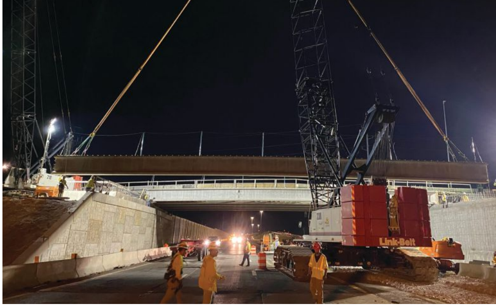
C. W. Matthews Contracting Co. Inc. sets a precast, prestressed concrete girder for the Interstate 75/Interstate 24 Interchange project in Tennessee. Several nighttime roadway closures were required for setting the girders at this and other overpasses on the project.
