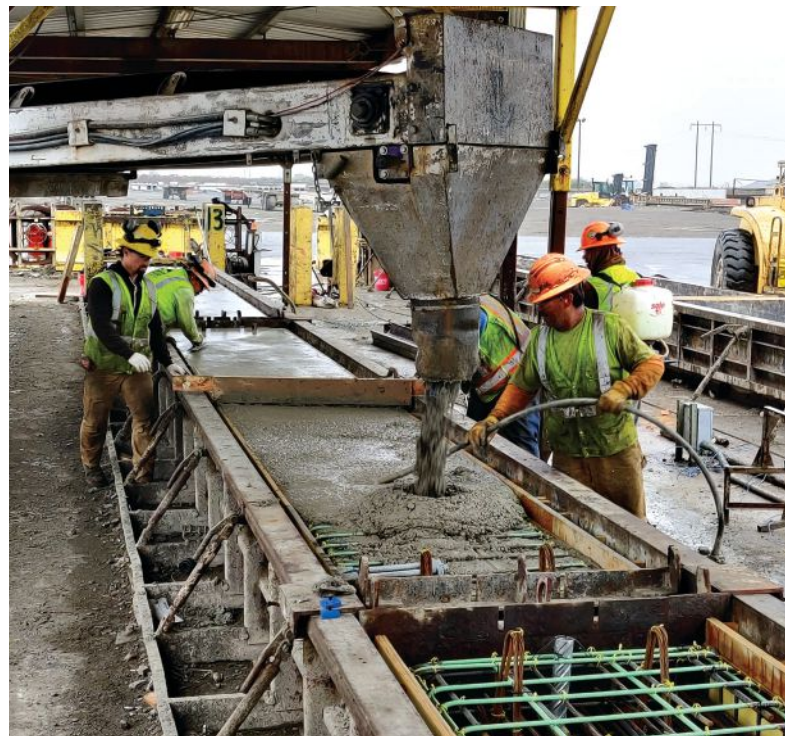
Figure 3. Concrete with 0.1% cellulose nanocrystals being placed, vibrated, and finished in the prestressed concrete girder formwork. Photo: Oregon State University.
