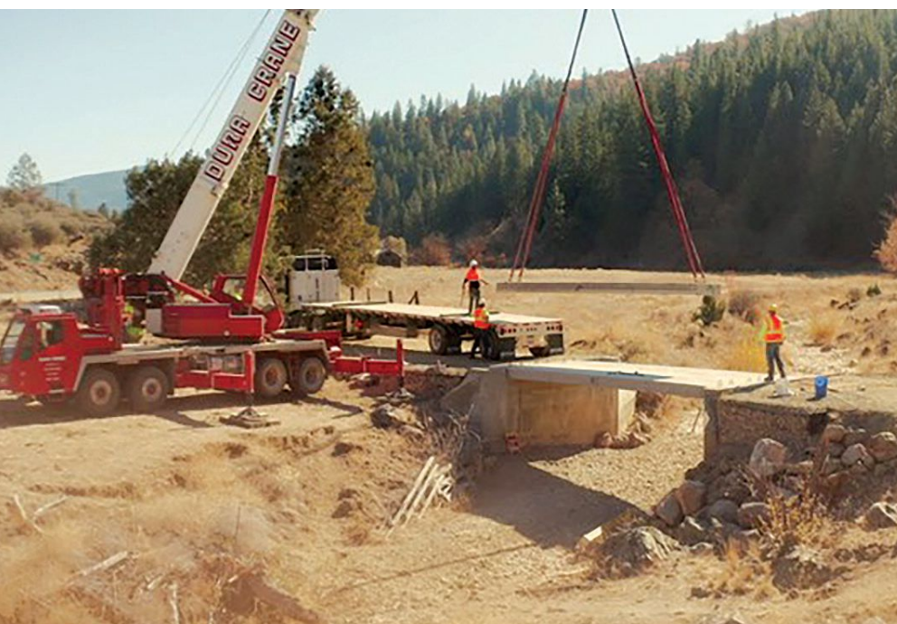
Figure 4. Successful installation of the prestressed concrete slab girders. The installation was performed using county personnel. Photo: Inland Films.
