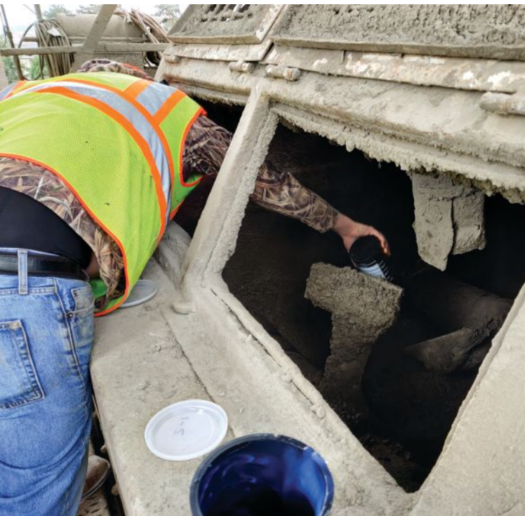
Figure 2. Addition of 0.1% cellulose nanocrystals through the observation hatch of the mixer as the concrete was being batched. Photo: Oregon State University.
