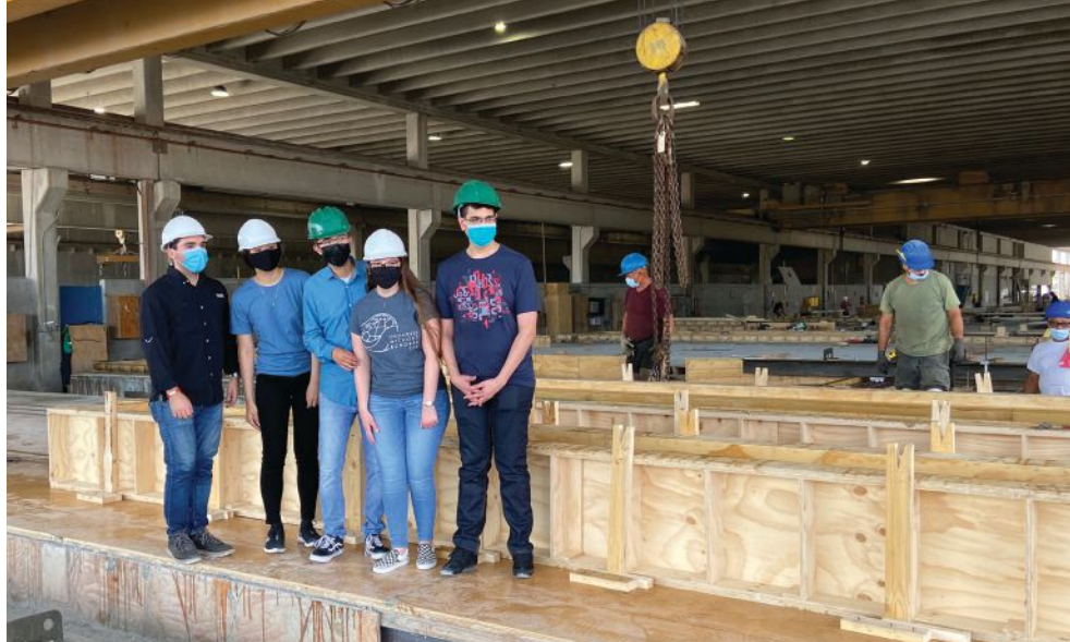
A group of students from Florida International University casting their beam at Coreslab Structures (Miami) Inc. for the 2020–2021 PCI Big Beam Competition.
