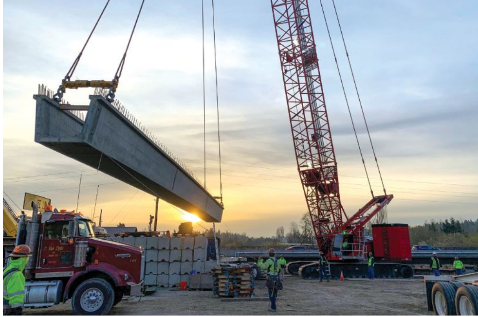
Installing one of the precast, prestressed concrete tub girders. The typical girder is 110 ft long and weighs 165 kip. Photo: Jacobs.
