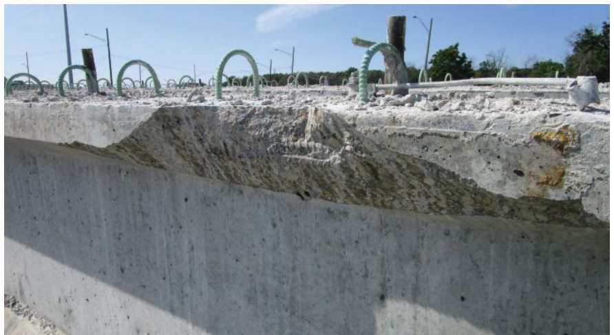
Figure 1. The top flange of this concrete girder was damaged during demolition. If the girder is to remain, it must be repaired. Photo: Collins Engineers.
