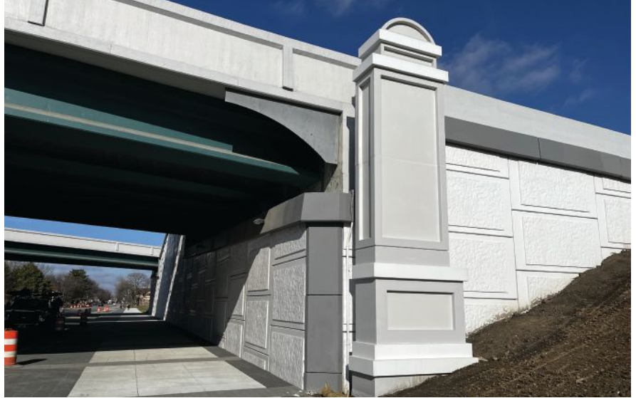
A component of the project's aesthetics and enhancements implementation plan is the placement of precast concrete corner monuments ranging from 22 to 38 ft in height. Here, a decorative monument is located adjacent to mechanically stabilized earth abutment walls. Photo: Janssen & Spaans Engineering.
