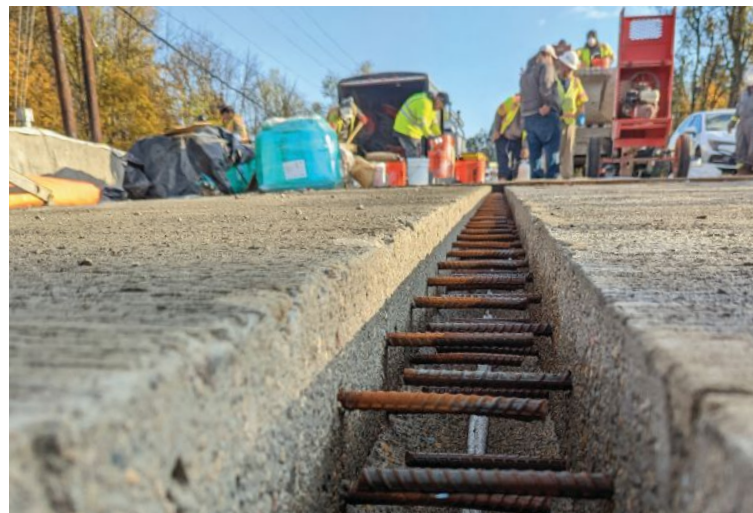
Figure 4. The contract specifications required an exposed-aggregate surface finish in the keyway pocket of the closure pour. The bottom of the keyway pocket is sealed to prevent the fluid ultra-high-performance concrete from seeping.
