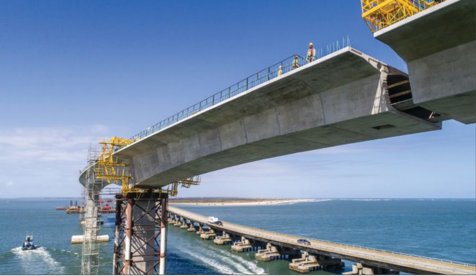
The navigation unit of the Marc Basnight Bridge, Outer Banks, N.C., is a 3550-ft-long, 11-span, continuous post-tensioned concrete segmental structure. It received the 2019 American Segmental Bridge Institute Award of Excellence. Photo: HDR.
