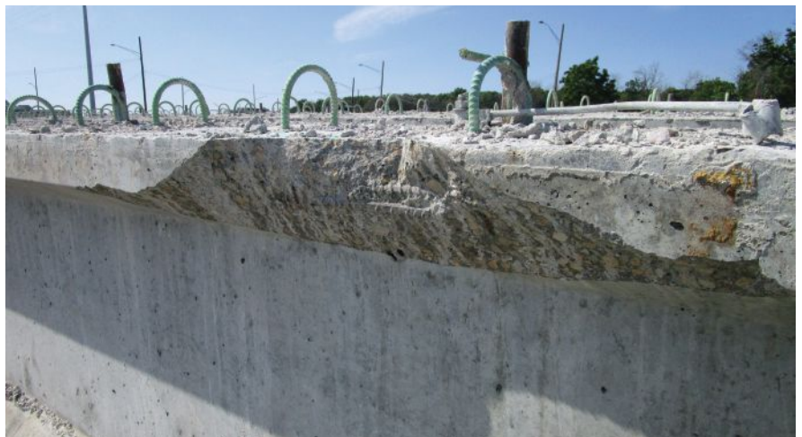
Figure 1. The top flange of this concrete girder was damaged during demolition. If the girder is to remain, it must be repaired. Photo: Collins Engineers.
