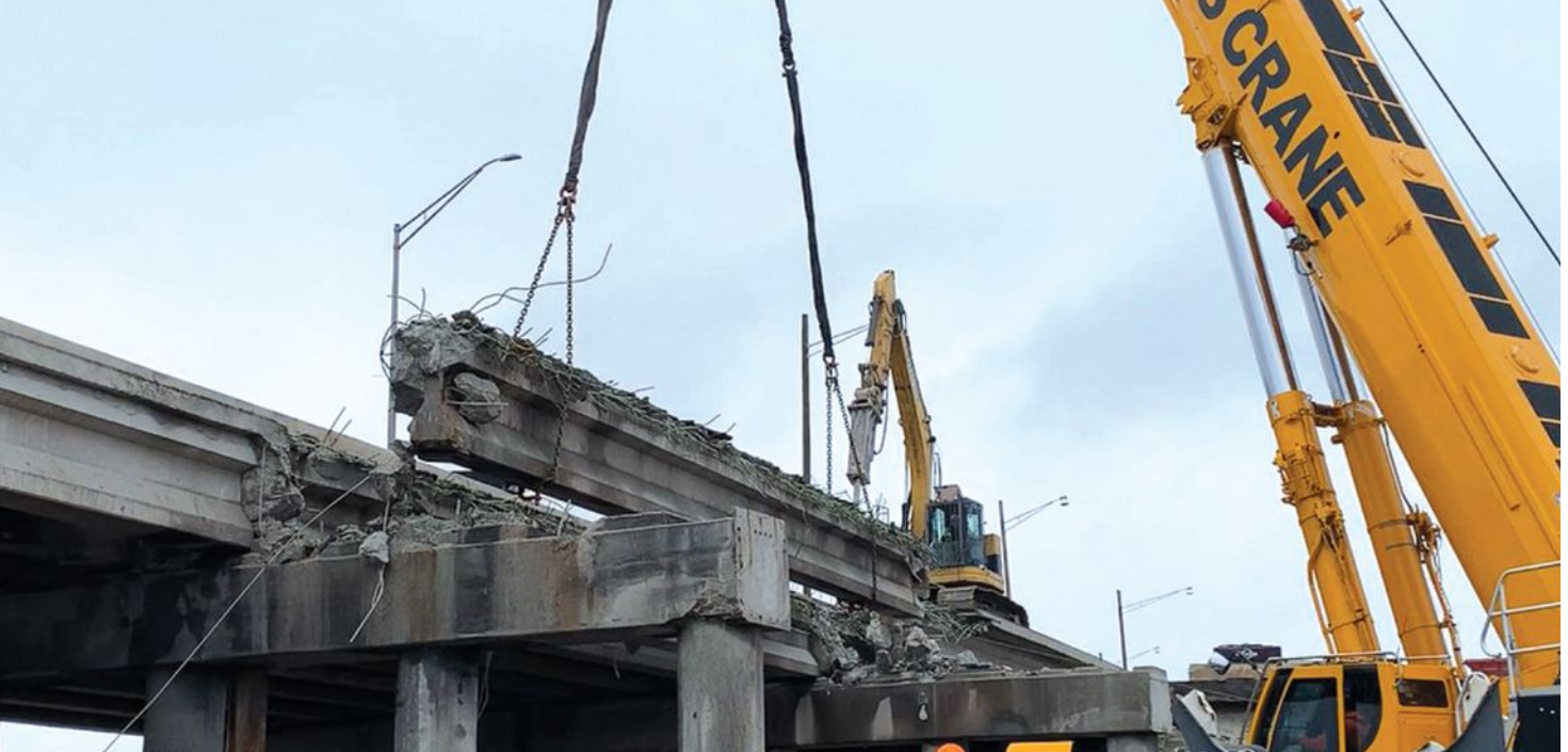
Figure 4. During demolition of a bridge superstructure, a prestressed concrete girder is removed using a single-crane pick. The demolition engineer should verify the proposed lifting configuration to ensure stability of the girder during its removal. Photo: Collins Engineers.
