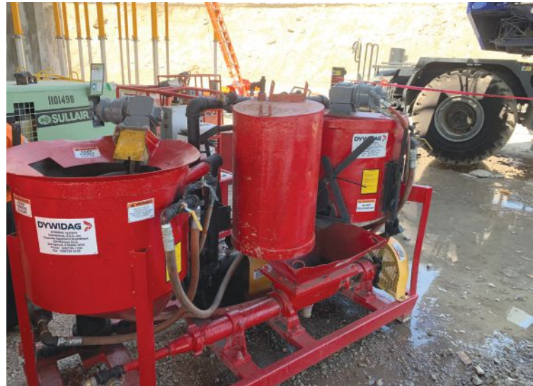
A colloidal grout mixer was used to prepare the grout. The tendon grouting was performed by certified personnel in accordance with Post-Tensioning Institute/American Segmental Bridge Institute grouting specifications.
