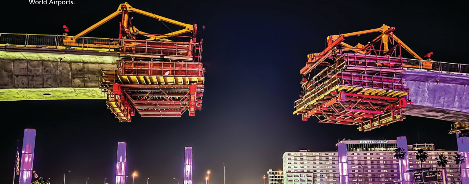
Night view of form travelers being used during concrete segmental construction of the 212-ft span over Sepulveda Boulevard in Los Angeles, Calif. Several spans use post-tensioned box girders (see the Fall 2023 issue of ASPIRE ® for details). Photo: Los Angeles World Airports.
