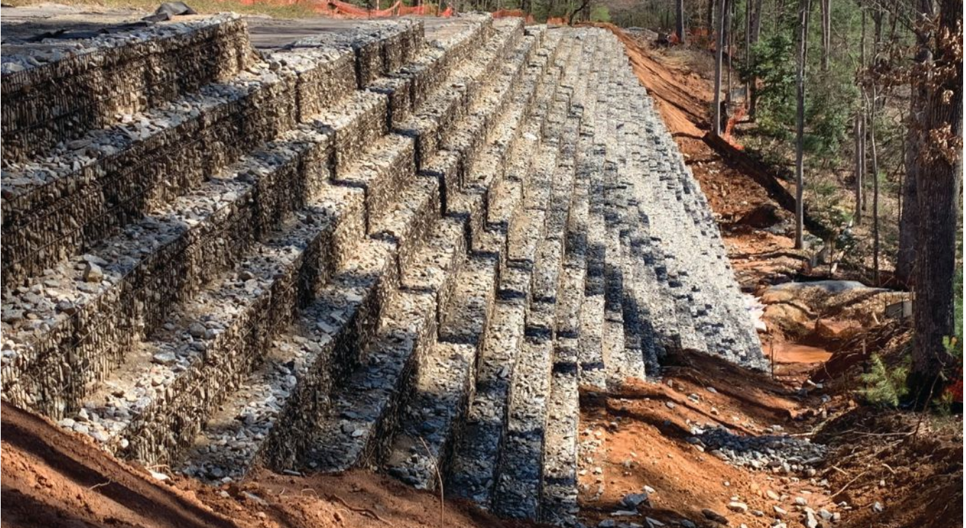
The reinforced-soil retaining wall at the Abutment 2 approach will have native grasses growing on the gabion baskets.
