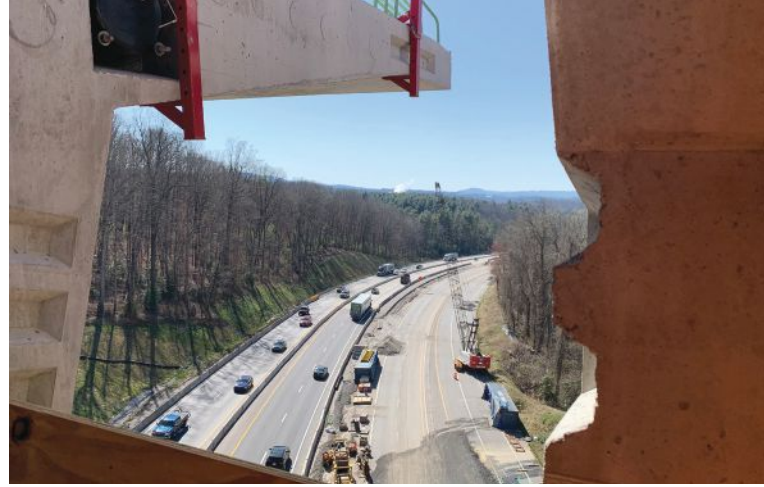
View of Interstate 26 through the main-span closure pour opening. The shear keys on the precast concrete segments are visible on the left and right sides of the photo.
