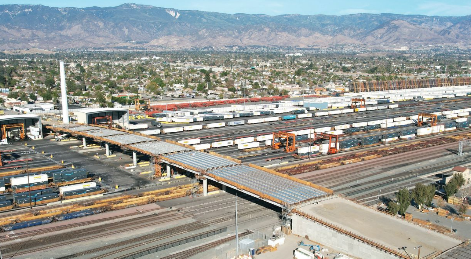
The new seven-span Mount Vernon Viaduct bridge and the one-span 3rd Street crossing use precast, prestressed concrete girders. Photo: Dany Schimpf Photography.
