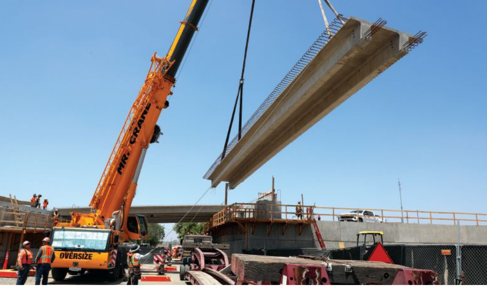
Setting of a prestressed concrete Northeast Extreme Tee (NEXT) girder at the 3rd Street overcrossing. The shallow 28-in.-deep NEXT girder is used to provide the 15-ft minimum vertical clearance. Photo: Dany Schimpf Photography.
