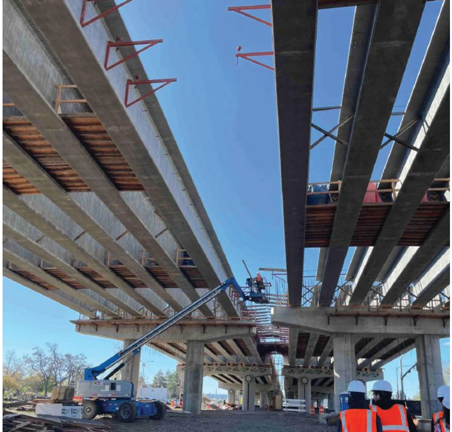
View from beneath the erected WF83G pretensioned concrete girders. Photo: Kuney Construction.
