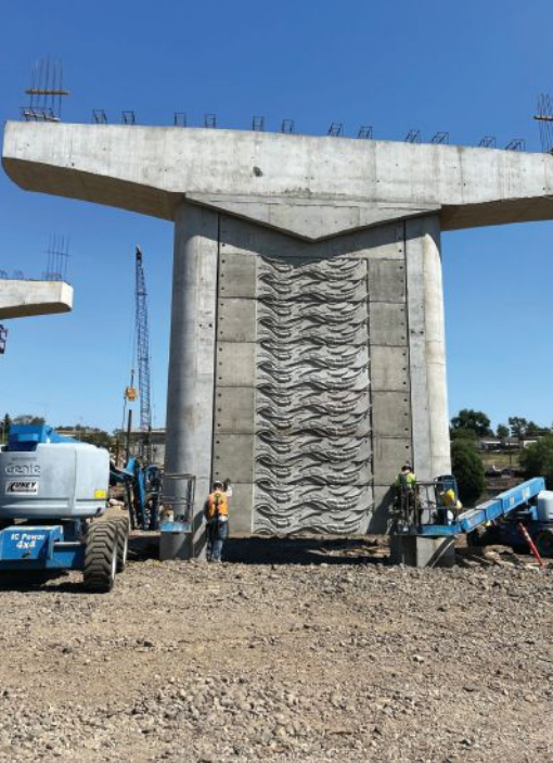
The cast-in-place concrete pier is a two-column structure with decorative precast concrete panels to give the illusion of a single-column pier. The panels will receive a base coat of gray pigmented sealer, and some areas of the concrete texture will be enhanced with accent colors. Photo: Kuney Construction.
