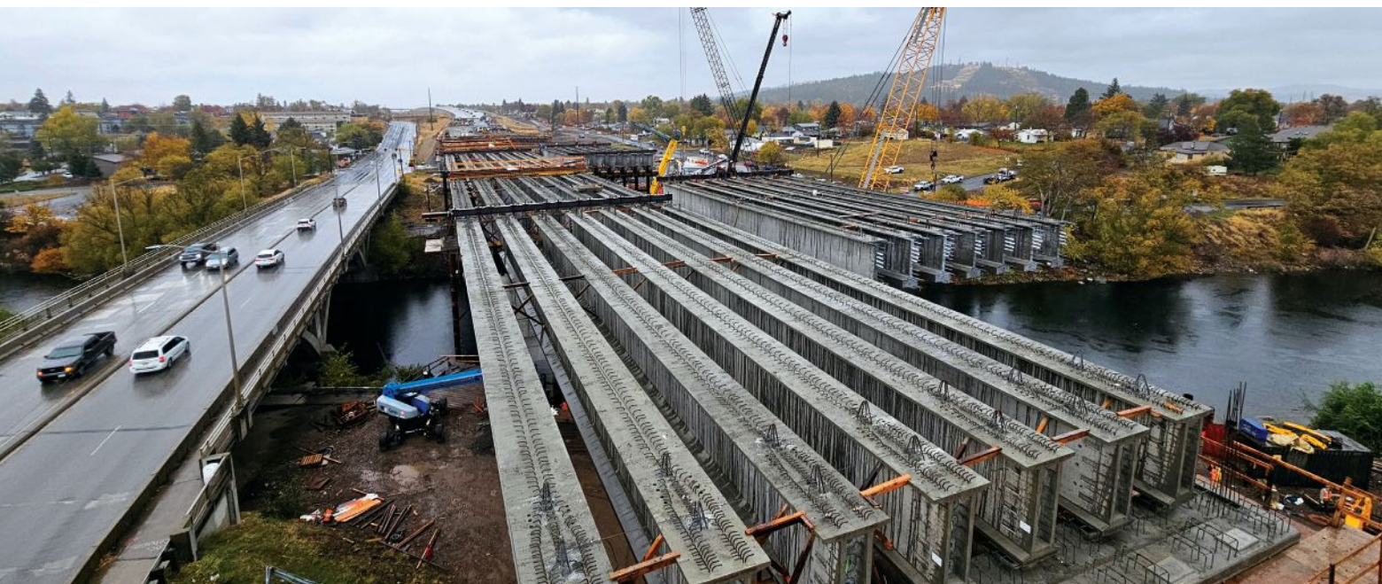
The girder lines of the southbound bridge are erected and ready for installation of post-tensioning. Photo: Knife River Prestress.
