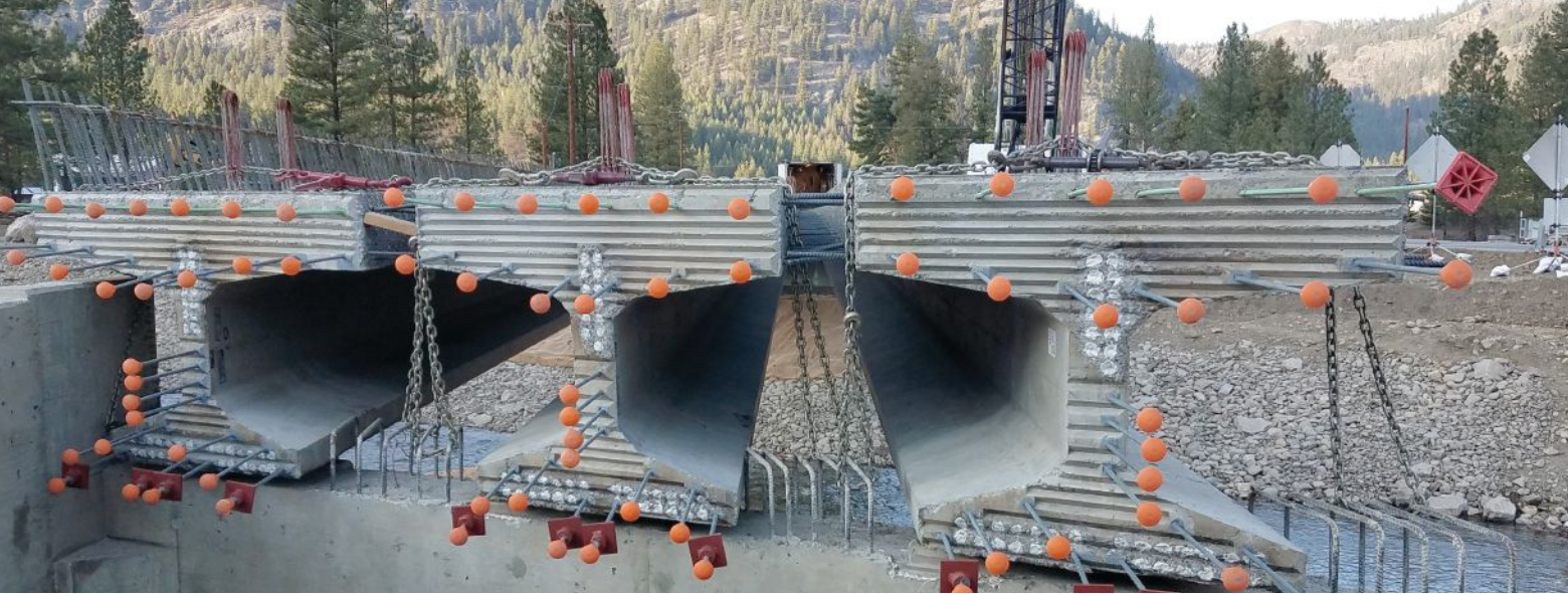
For the replacement of the San Poil bridge, the Washington State Department of Transportation used wide-flange deck girders with a thicker than standard top flange. The prestressed concrete girders eliminated the need for deck formwork. Ultra-high-performance concrete was used in the top-flange connections between adjacent WF39DG girders.
