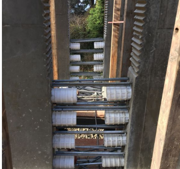
The crossing of U.S. Route 101 over Steamboat Creek used spliced, post-tensioned precast concrete girders and was the first Washington State Department of Transportation project to use plastic ducts in prestressed concrete girders. The high-density polyethylene ducts are intended to protect tendons from corrosion. Shown here is a closure joint before the duct couplers, additional reinforcement, and post-tensioning are installed and concrete cast.
