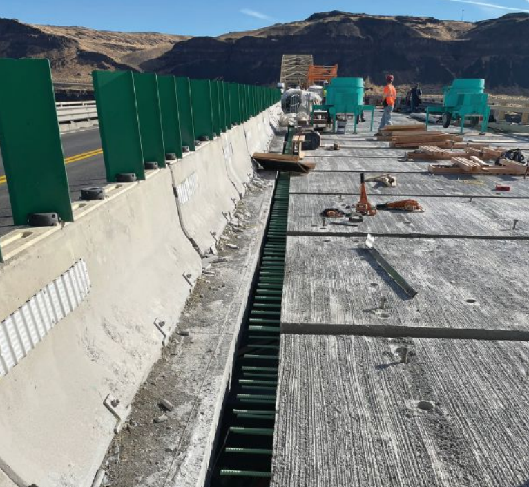
The replacement of the existing bridge deck on the Interstate 90 Vantage Bridge aims to maintain the structural integrity and extend the life of the bridge. While allowing traffic on adjacent lanes, construction is currently underway using precast concrete bridge deck panels and ultra-high-performance concrete in the longitudinal and transverse keyway joints.
