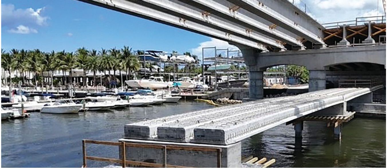
The Florida slab beams, piles, and bent caps of a low-level observation deck at the U.S. Route 1 bridge replacement in Jupiter, Fla., have carbon-fiber-reinforced-polymer prestressing strands and glass-fiber-reinforced-polymer reinforcement.
