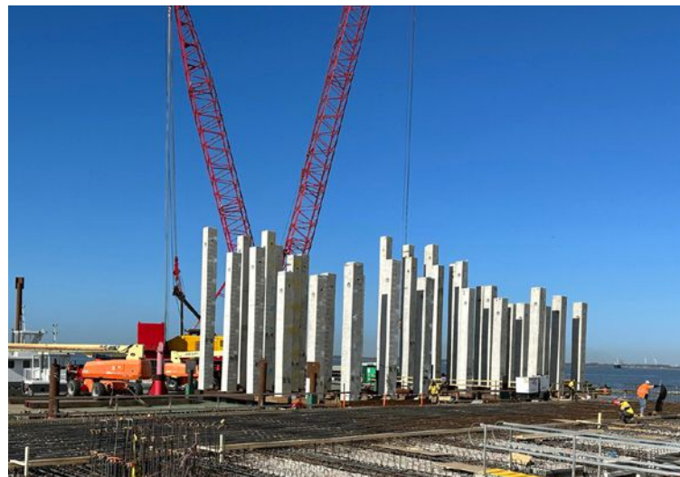
Photos: Jacob Ray (Moffatt & Nichol) and New Jersey Economic Development Authority (NJEDA) taken by Drone Deploy.
