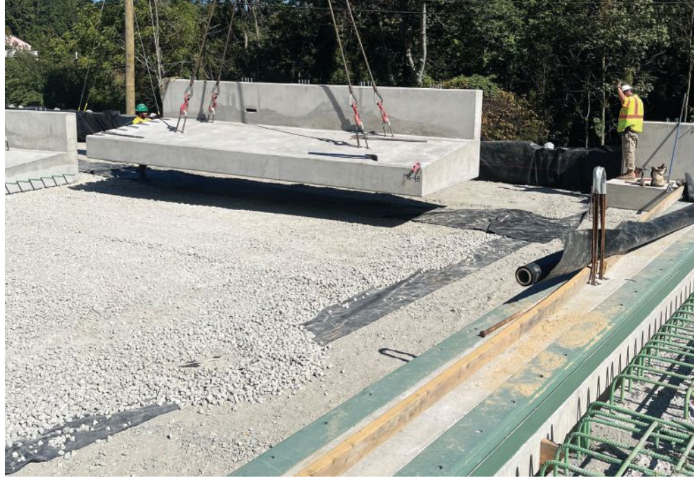
Moment slab segments were cast with the sleeper slabs to accommodate the transition from bridge barrier to guardrail.
