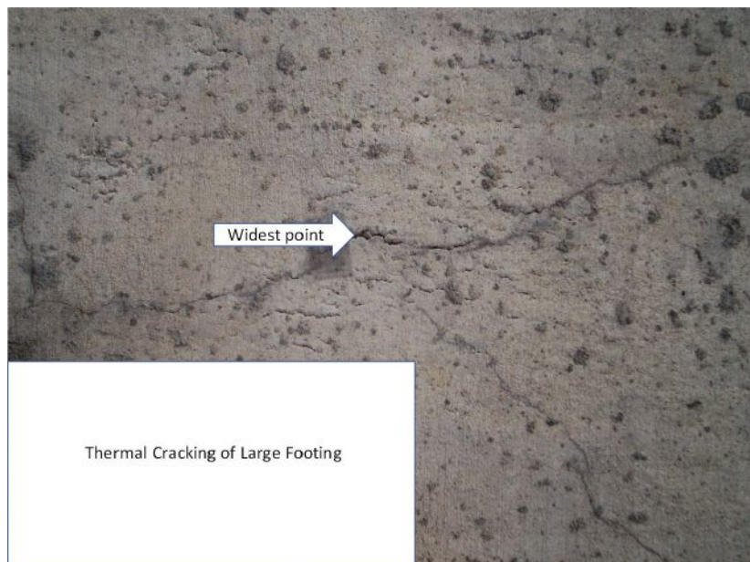
Figure 4. Cracking due to temperature gradients can be problematic with mass concrete placement. Figure: University of Texas at Austin.
