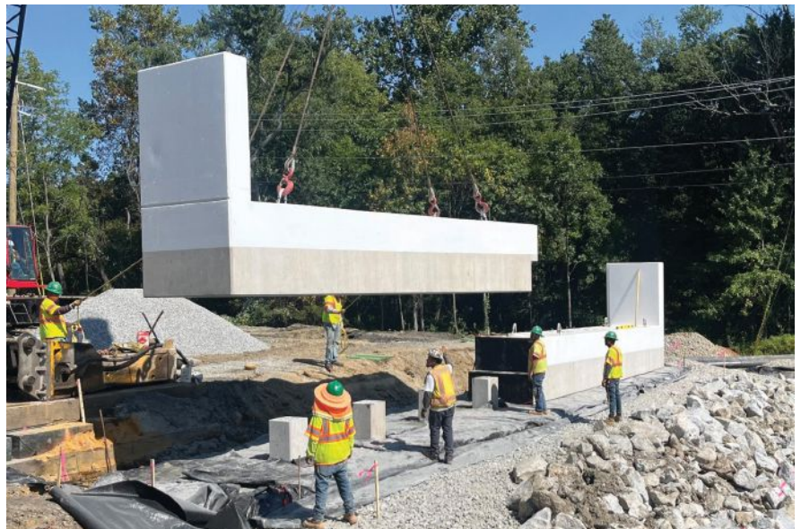
A precast concrete abutment segment is set into place over piles. Note the shiplap joint where two segments will be joined. All Photos: Delaware Department of Transportation.
