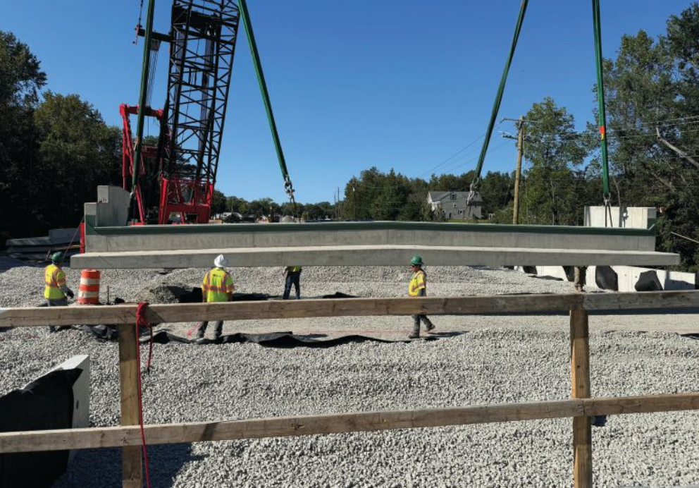
The 51-ft 6-in.-wide sleeper slabs were cast as a single precast concrete element and were connected using ultra-high-performance concrete closure joints.
