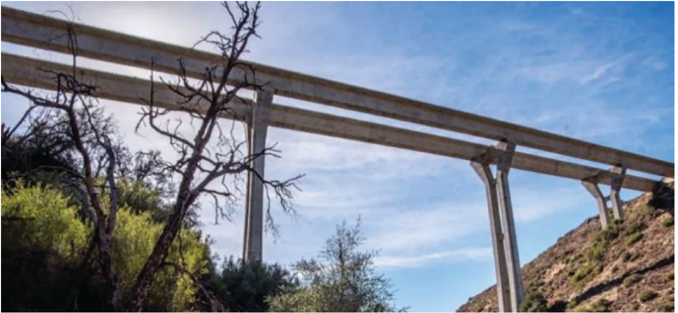
Figure 2. Pine Valley Creek Bridge in Pine Valley, Calif., is the first long-span concrete segmental box-girder bridge in the United States built using the cast-in-place balanced-cantilever method.
