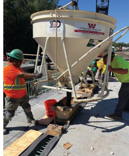
Workers place ultra-high-performance concrete (UHPC) from a concrete hopper into a longitudinal joint between adjacent decked bulb-tee beams. After the UHPC is placed, the joint is top formed and a pressure head system is created.
