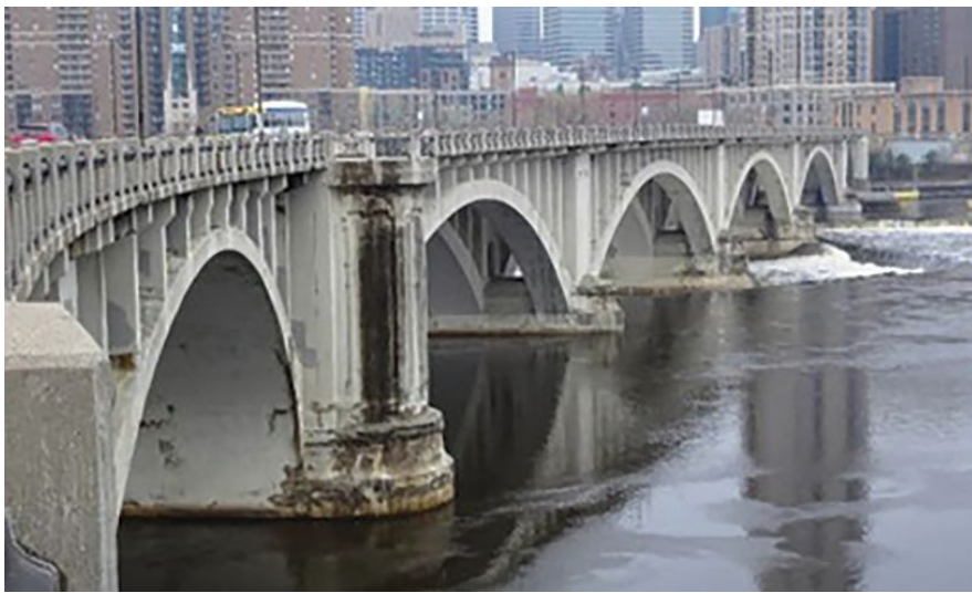
The upstream side of the historic Third Avenue Bridge in Minneapolis, Minn., is shown before rehabilitation was undertaken. Note the concrete deterioration in the pier bases and arches. Photo: Wiss, Janney, Elstner Associates.
