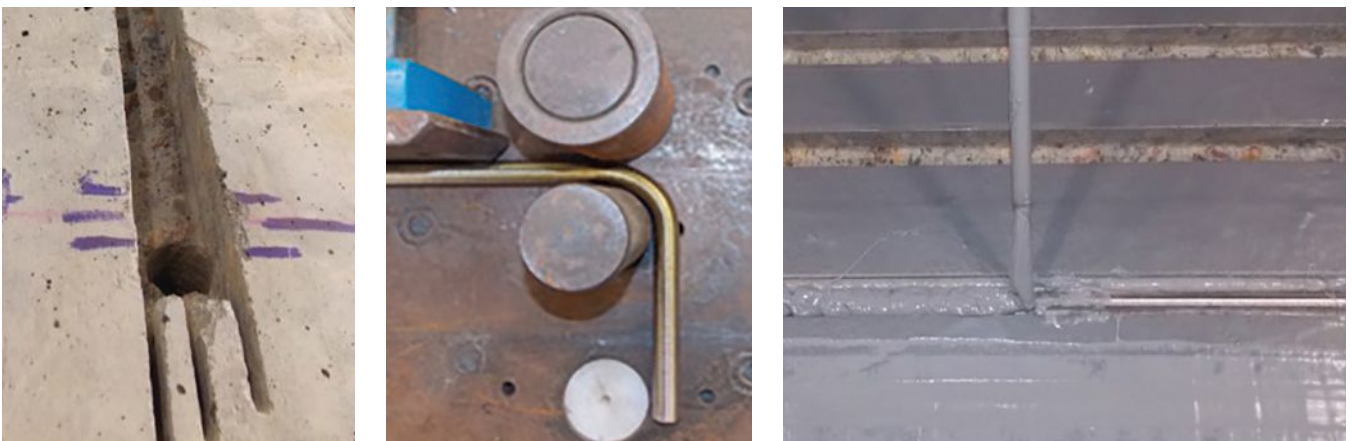
Figure 1. Installation of near-surface-mounted titanium alloy bars (TiABs): Saw-cut groove in cover concrete and hammer-drilled hook anchorage hole into core (left); bending of TiAB with 90-degree hooked ends (center); TiAB is installed and grooves filled with structural epoxy with exposed surfaces taped for a clean surface finish (right). Photo: C. Higgins, Oregon State University
