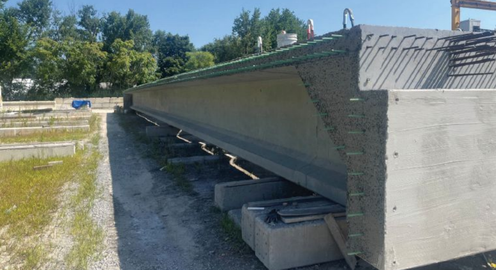
An adjacent decked bulb-tee beam is staged in the precaster's yard. The precast concrete interface that will form the side of the longitudinal joint has a roughened concrete surface and reinforcement that will project into the joint to help the UHPC bond to the precast concrete beam.
