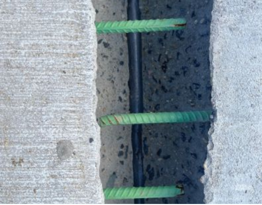
A close-up view of the approach slab joint showing the noncontact lap splice between the precast concrete elements. Backer rod is used to create a watertight seal and prevent ultra-high-performance concrete leakage.
