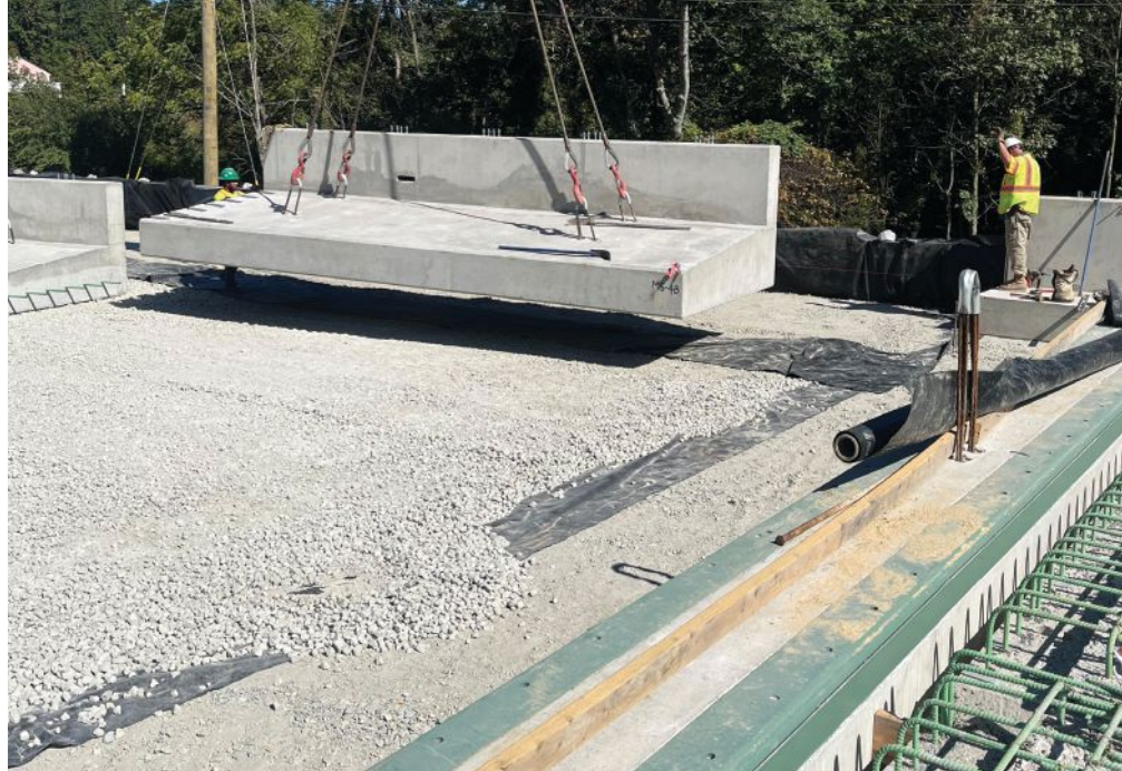
Moment slab segments were cast with the sleeper slabs to accommodate the transition from bridge barrier to guardrail.
