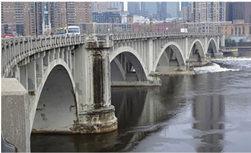
The upstream side of the historic Third Avenue Bridge in Minneapolis, Minn., is shown before rehabilitation was undertaken. Note the concrete deterioration in the pier bases and arches. Photo: Wiss, Janney, Elstner Associates.
