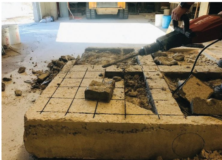
Figure 2. Concrete removal method 4 uses the most saw cutting of the four tested methods to reduce the jackhammering time. The concrete removal time, equipment usage, and labor required for partial-depth concrete deck repairs were compared for each method.
